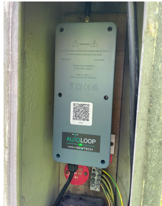
Autoloop installed in a lighting column
